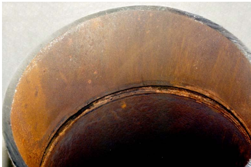
Figure 9 Weldment Corrosion in a Condensate Line (CO 2 system)
