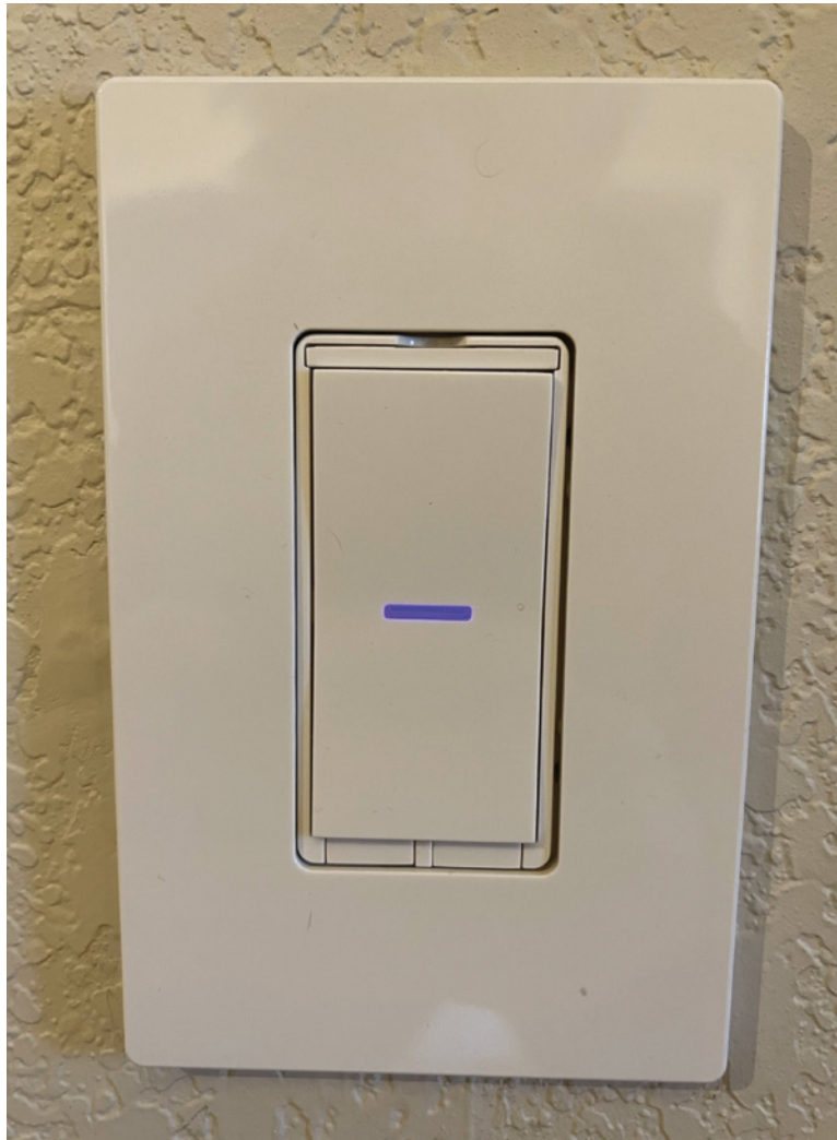
FIGURE 15.19 Internet-enabled light switch
